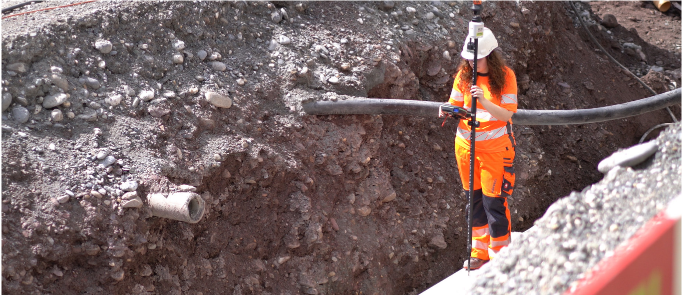
Figure 5: Speed up work using Tilt Compensation and simultaneously increase the operator's safety at challenging site conditions.
